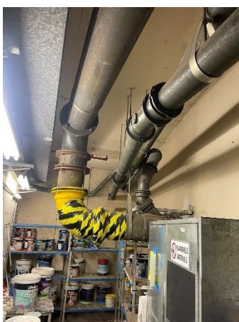
Existing Mild Steel sewer drainage.
