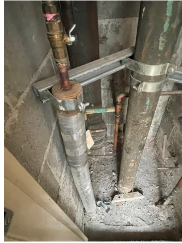
Existing Hot Water services pipework.
