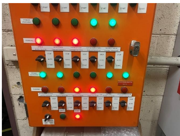
Figure 15: Existing Fire Fan Control panel (FFCP).
