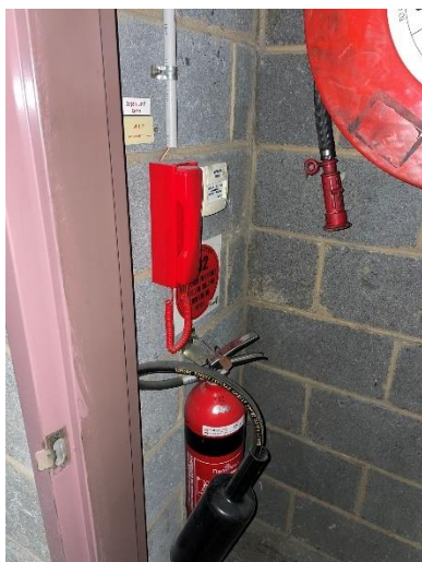
Figure 18: WIP/ECP points within cupboard.
