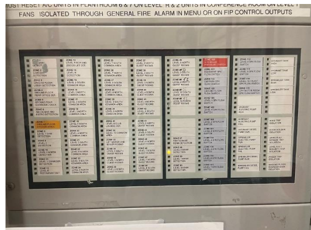
Figure 14: Existing addressable fire indicator panel inc. FFCP
