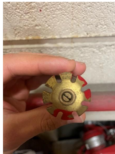
Figure 8: Sprinkler heads example and sprinkler pipes
