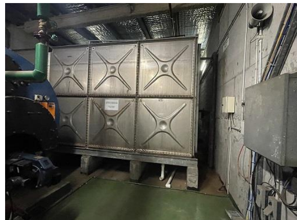
Existing Combined CW. & FH water storage tank.
