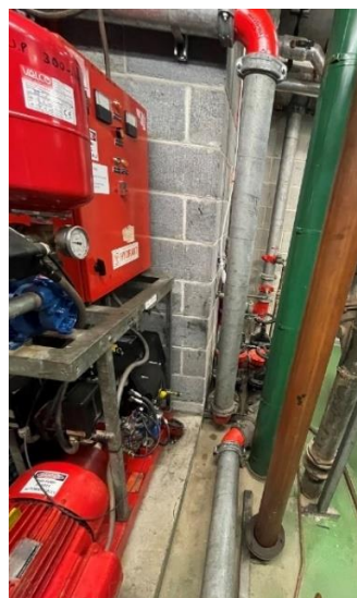
Figure 2: Existing Diesel/Electric Hydrant pump
