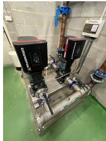
Existing CW. booster pumps.
